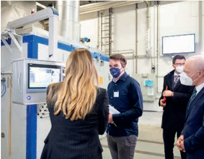
The monitors next to the TopChem production system show all the key furnace parameters such as temperature distribution and air volume flows in real time.
