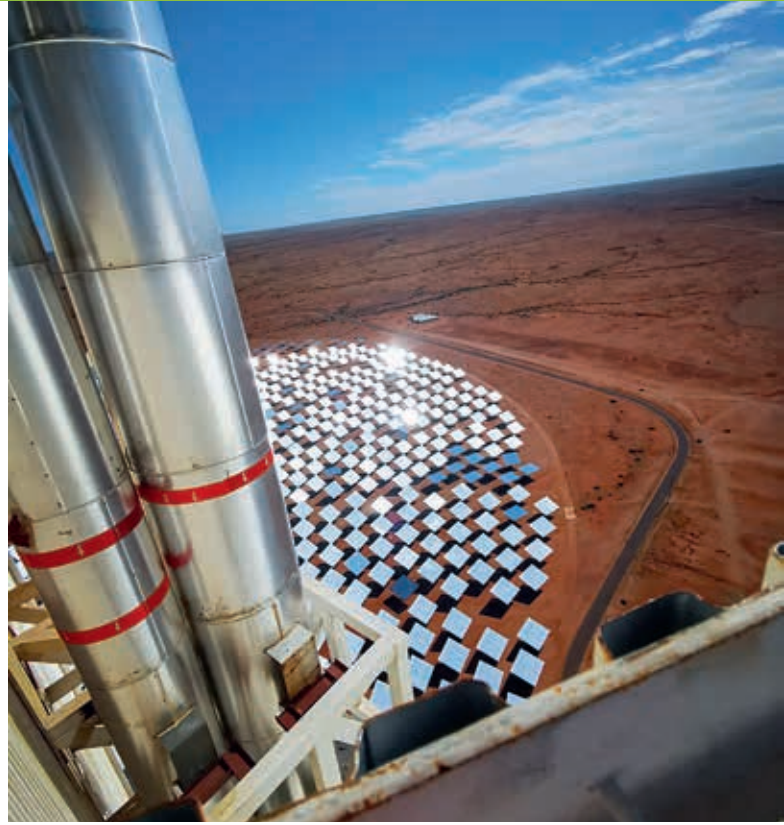
Khi Solar One's solar tower
