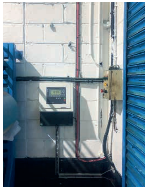
Air compressor control unit in new location
