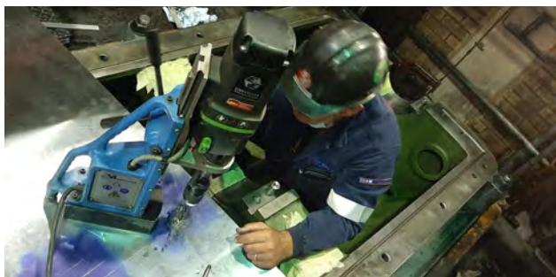
Technician preparing the Mounting Plate to ensure machine is set up Level with all surface
